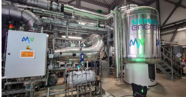
Figure: River heat pump from MVV Energie AG in Mannheim | © MVV Energie AG
