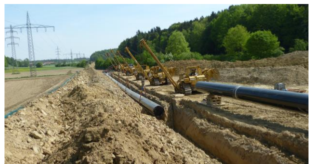
Figure: Construction of the MONACO gas transport pipeline: Caterpillars lowering the pipe into the trench | © bayernets GmbH
